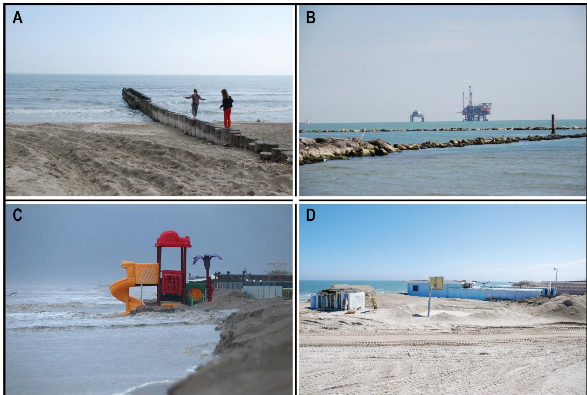
Figure 12: A and B) Coastal protection works in the Ravenna coast with parallel and transversal groynes; C and D) fixed structures on the beach in the Ravenna coast damaged by the winter storms.
