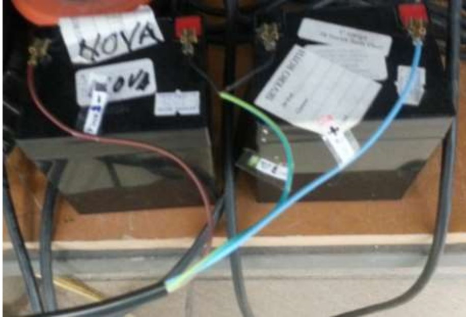
Figure A.26: Two parallel-connected 12 V batteries. The brown cable is connected to the negative pole of the circuit, the blue cable to the positive, and the green-yellow cable connected to remaining poles of the batteries, creating a real ground
