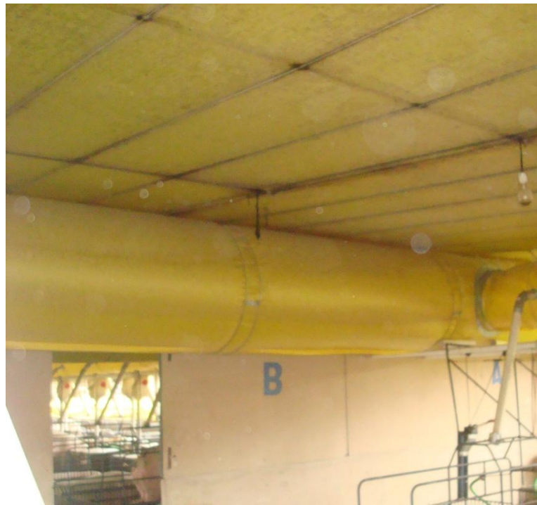
Figure 3 - Curtains tubular plastic (duct) connected to the system cooling air
