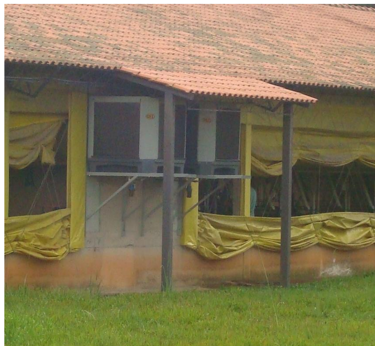
Figure 2 - Cooling System air (evaporative) located on the outside of the farm
